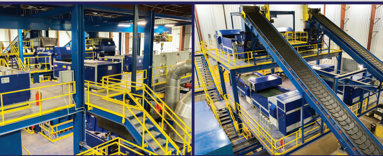
20tph ASR Plant in Milwaukee, Wisconsin
